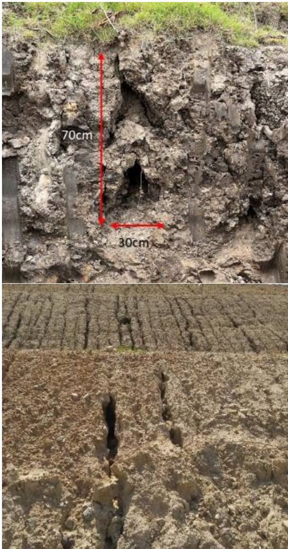
Figure 5 Dribble pattern and pothole in d/s slope of the dam
