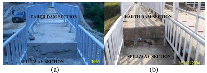
Figure 8 The settlement of the earth fill (Photo by RID): (a) 2003; (b) 2004
