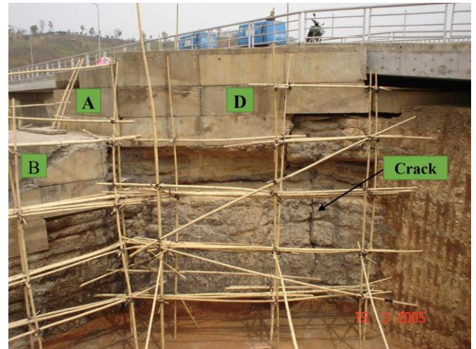
Figure 12 Crack in RCC Block D (Photo by RID, 2005)
