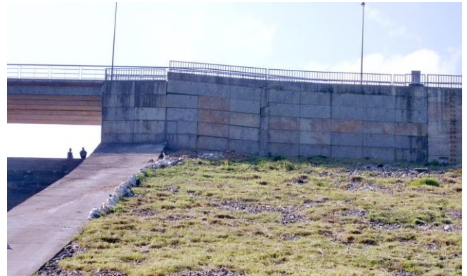
Figure 7 Elevation of RCC Block D and differential settlement at left bank (Photo by RID)
