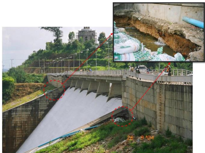
Figure 5 Leakage observed at the joint between RCC and earth fill dam; the differential settlement is clearly seen (Photo by RID)
